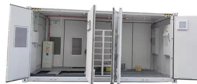
1075KW HH ESS
